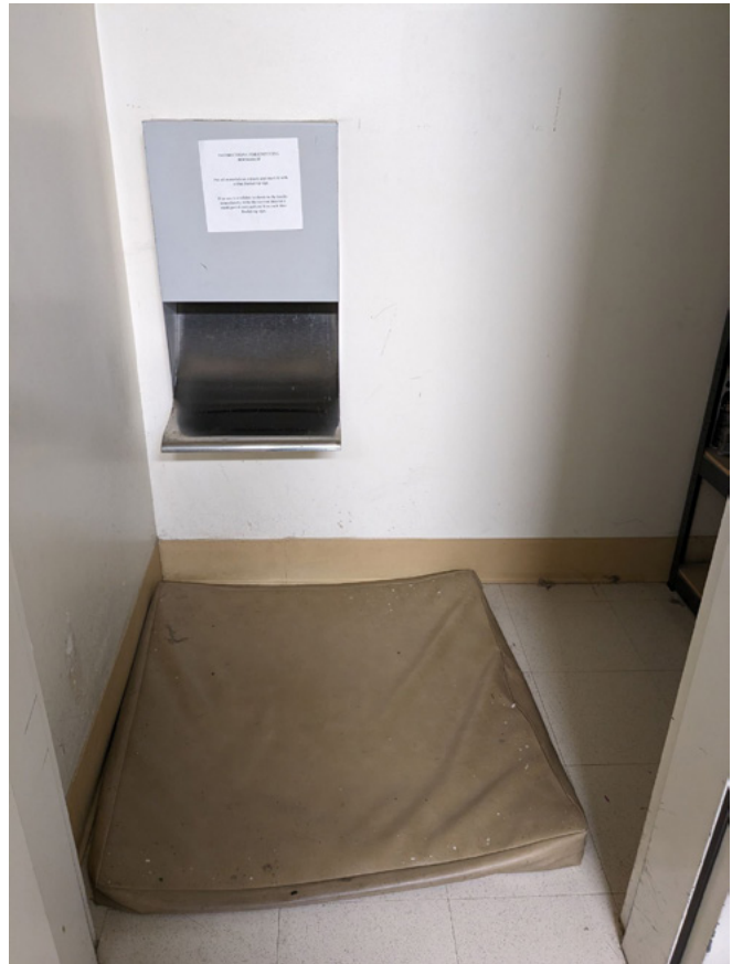
An example of adequate clearance not being provided for a bin below the book drop. A cushion was placed on the floor to receive the dropped books, which must be collected up by staff (an ergonomic issue).
